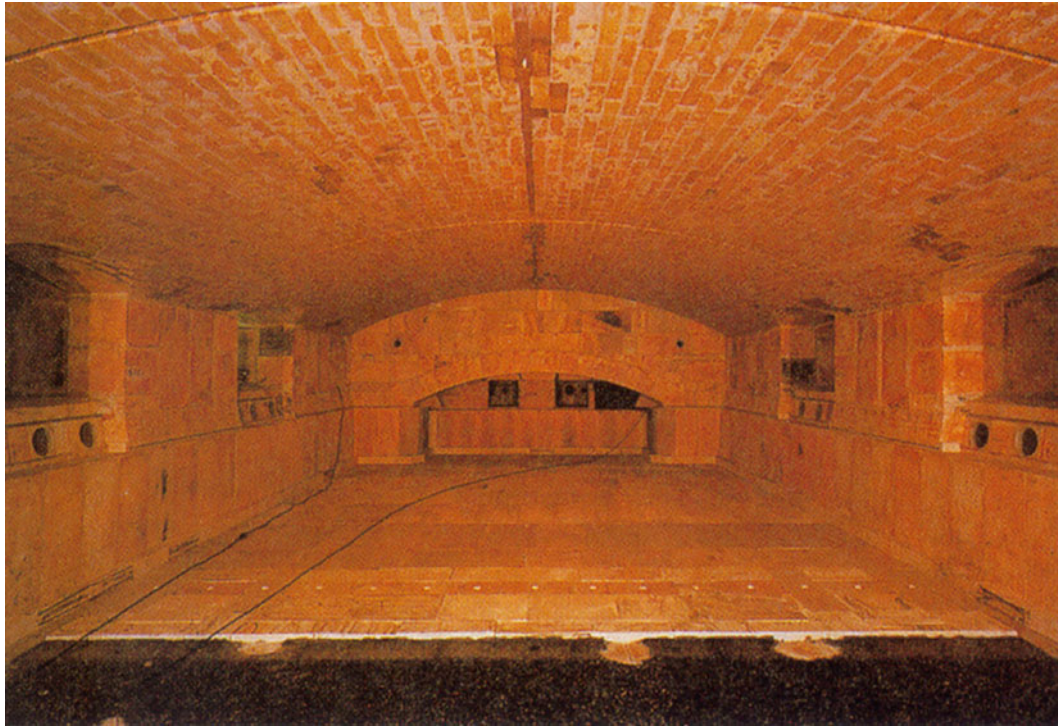
FIGURE 26.2. Inside a typical glass-melting tank.
