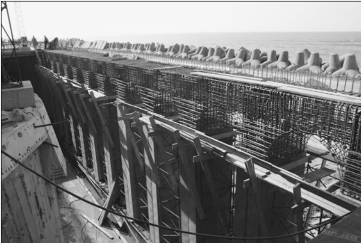
Reconstruction, using high-performance stainless steel reinforced concrete, of the 100 external combs supporting the peripheral slabs. The columns are called 'combs' because they have a wave-breaking effect. In the background you can see the sea and temporary dyke that was built to keep the construction site dry, as well as the tetrapods maintaining the dyke. (© Christine RAYNAUD - BTPM).
