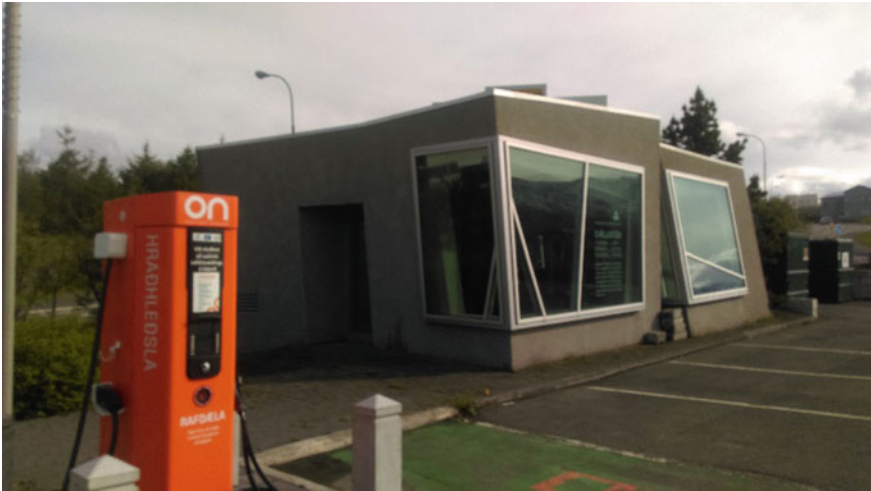
Fig. 21.6 Methane/biogas refilling station
