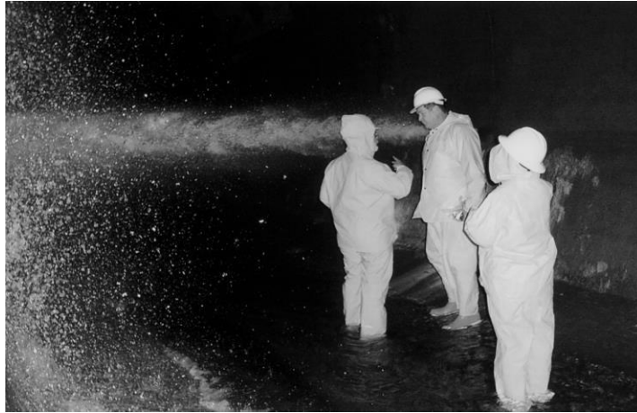
Fig.19: Encounter with underground water problem
